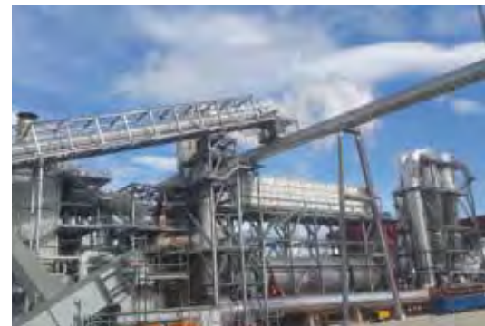
Energy plant and drum dryer
