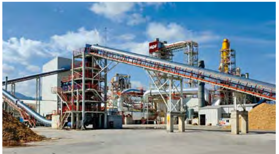
Conveyor and wood preparation technology in an MDF plant
