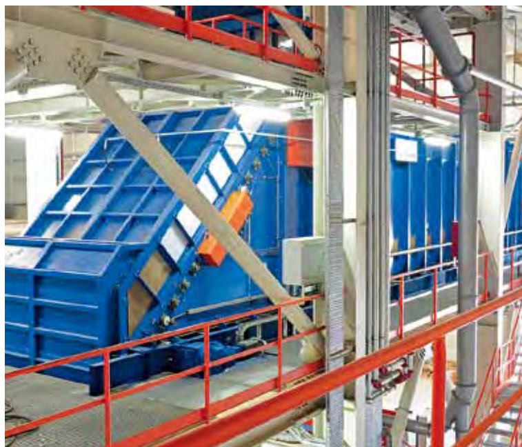
Fiber dosing bin
